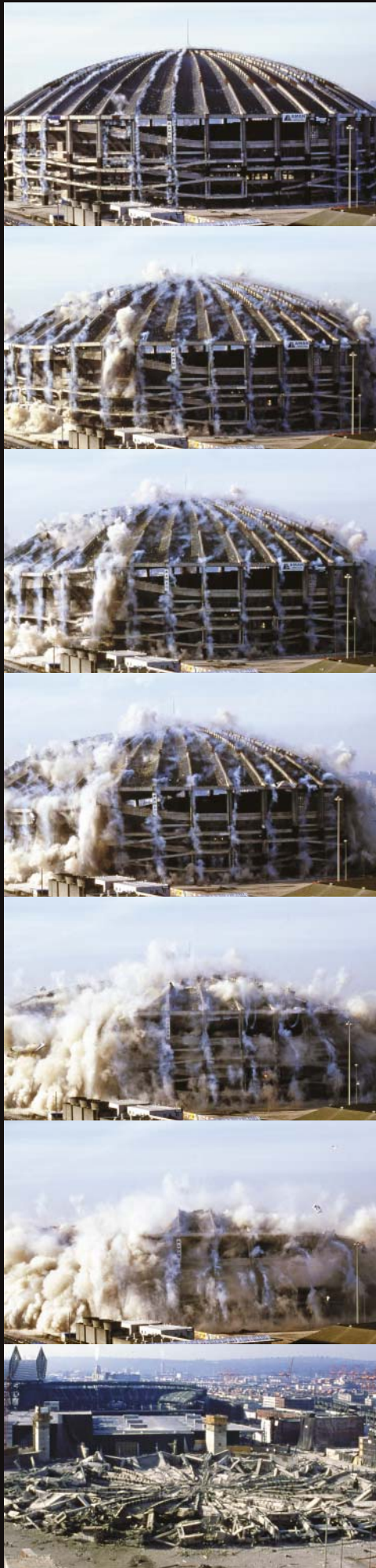
The Kingdom's unique post-tensioned construction to support the largest concrete dome on earth necessitated a whole level of dynamic control never needed on previous CDI projects. CDI needed to create controlled venting of millions of cubic feet of air from the structure to safely bring it down while preventing damage to 100-year-old historic structures directly across the street.
